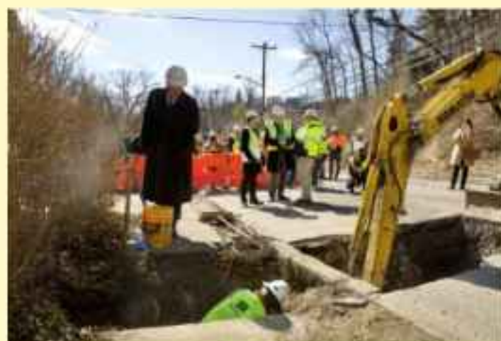
EPA Office of Water Deputy Assistant Administrator Bruno Piggot observes the 10,000th lead pipe replacement in Pittsburgh, Pennsylvania (PWSA, 2023c). Image source: PWSA
